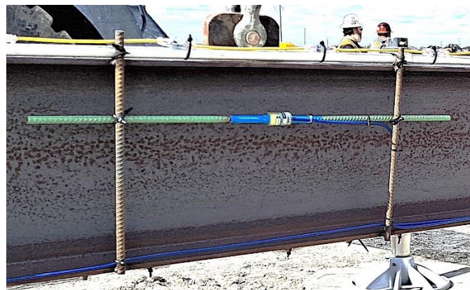
Fig. 3. Typical strainmeter installation.
