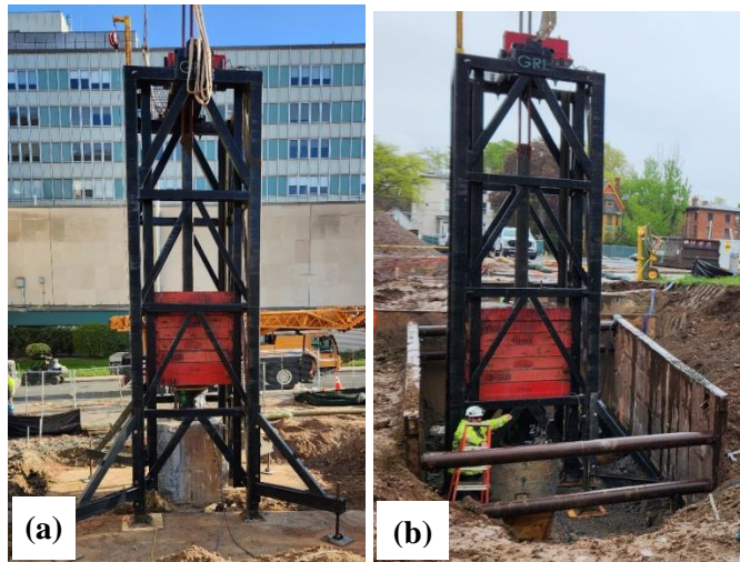
Fig. 3. Imagery of HSDLT on 3-foot-diameter caissons: (a) TS3-D1.0. (b) TS12-A3.2.
