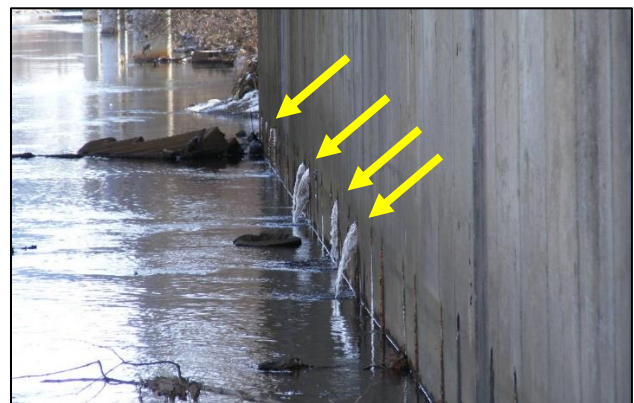
Photo 2: Constantly flowing forward abutment weep holes. Weeps are 3 feet above creek level and shown after 13 months of low rainfall.
