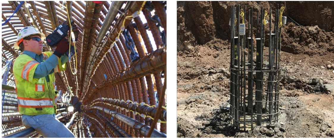
Figure 8. Thermal Wire cable attachment (left) and TAG and TAP-Edge Equipment (right).
