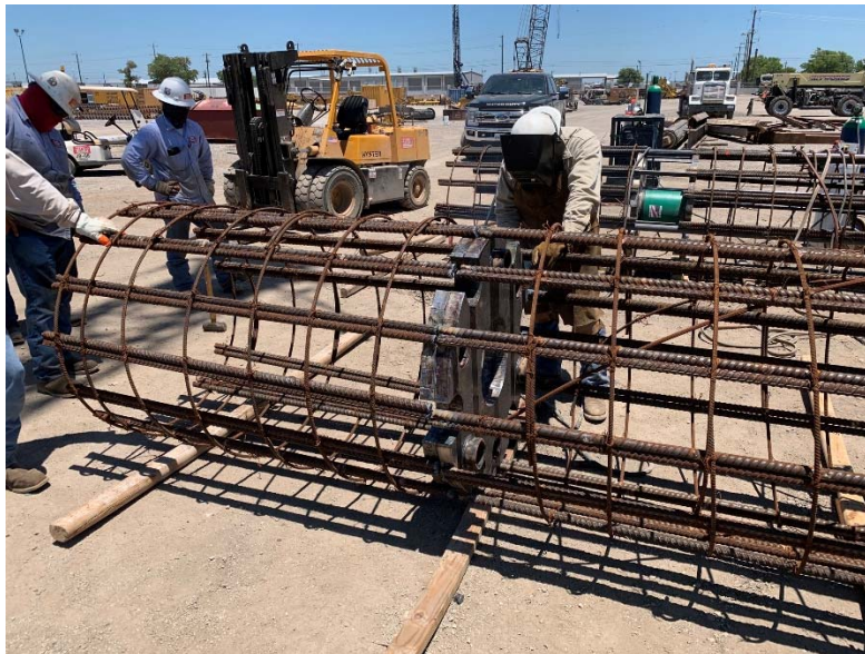
Figure 7. R-system installed within the rebar cage and at the geotechnical balance point
