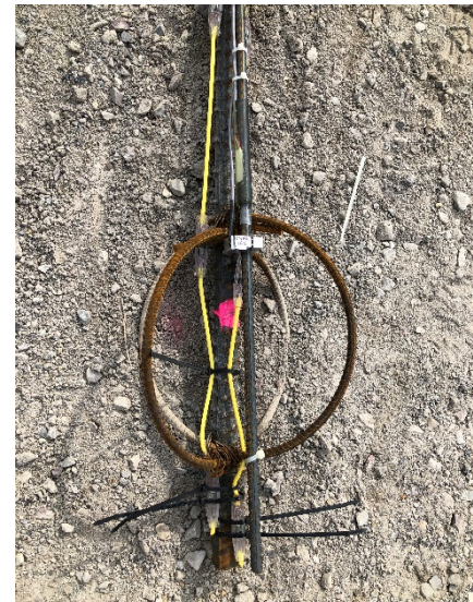
Figure 11: Center bar instrumented with sister bar strain sensor and Thermal Wire cable.
