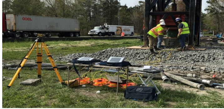
Figure 8: The crew is setting the drop height of the 16-ton ram; the force transducer is placed between the red ram and the pile top.
