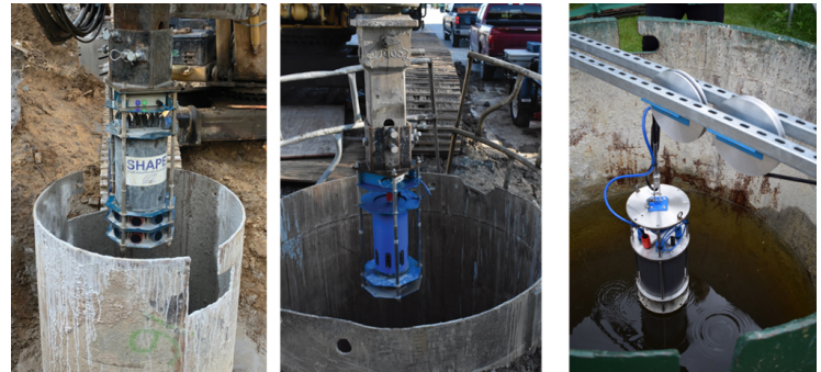
Figure 1. Kelly bar mounted SHAPE® (left) and SHAPE®-AIR (center) and winch-controlled SHAPE® with data transfer cable (right) testing drilled shaft excavations
