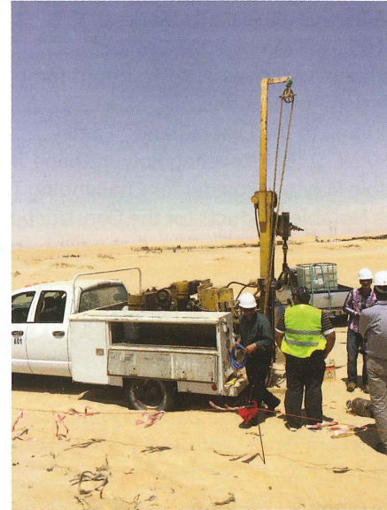
One of the recently calibrated Ayed Eid Al Osaimi Engineering Office SPT rigs
